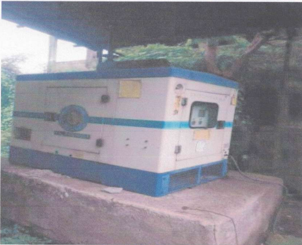
Generator 54 kw 15 KV
