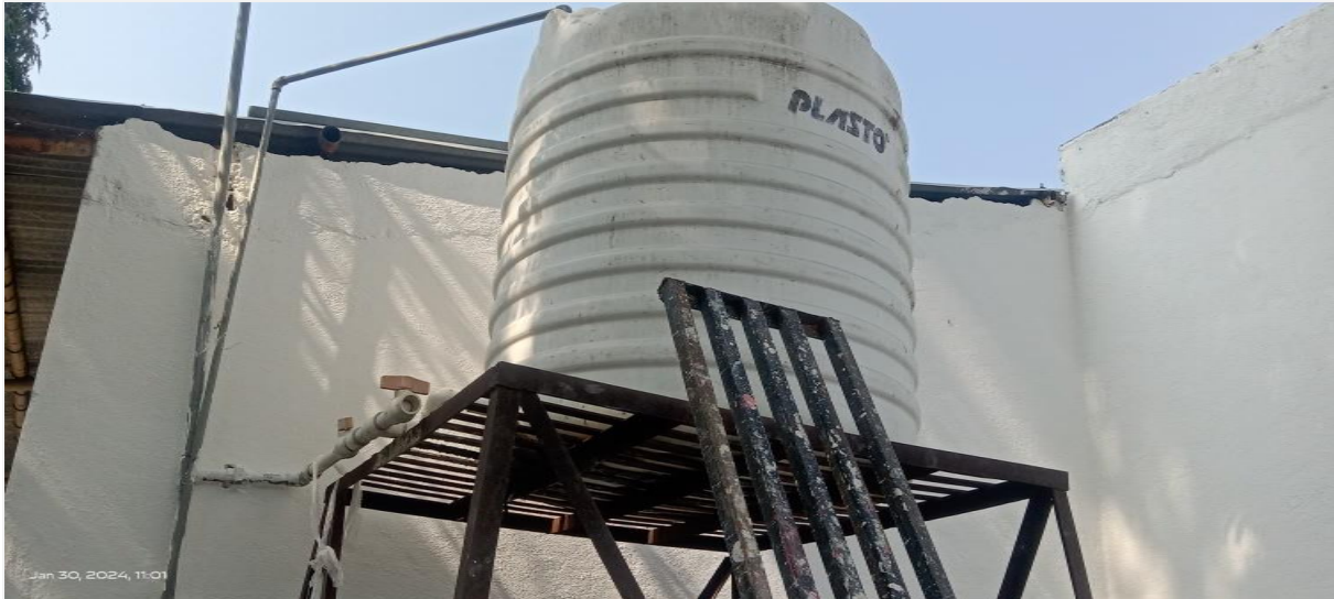
Plate 4: Water tanks on the rooftop
