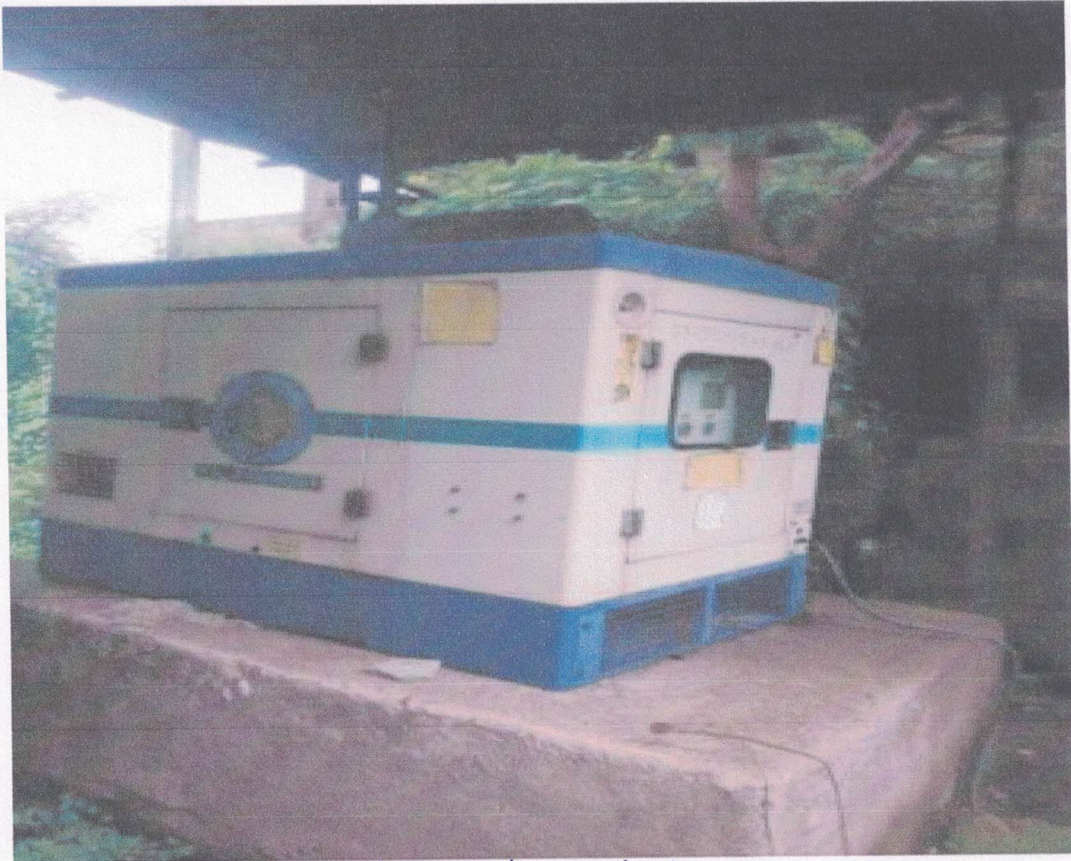
Generator set 15 KV
